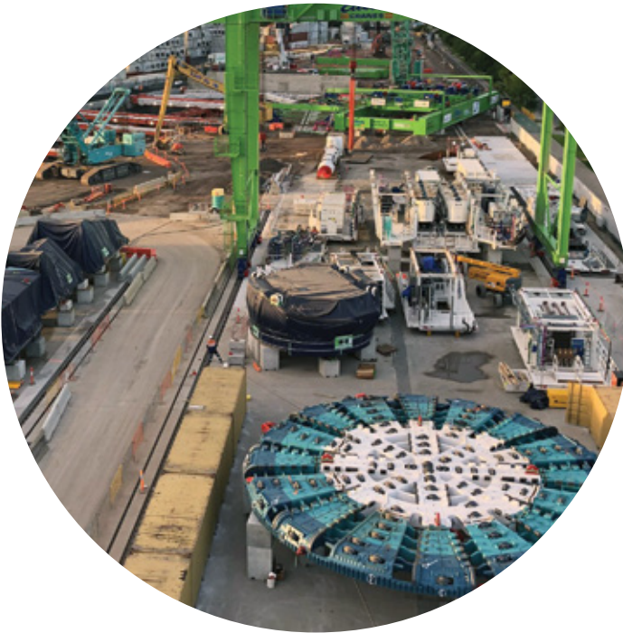
One of the giant tunnel boring machines being assembled to start tunnelling on the West Gate Tunnel Project
